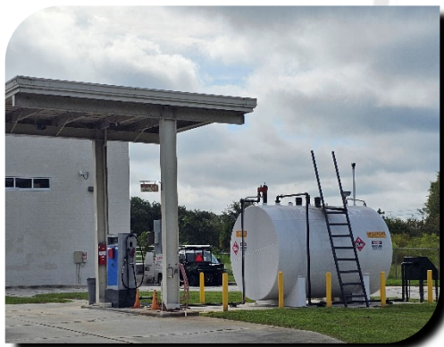
Picture 7: Fuel tank for fleet
